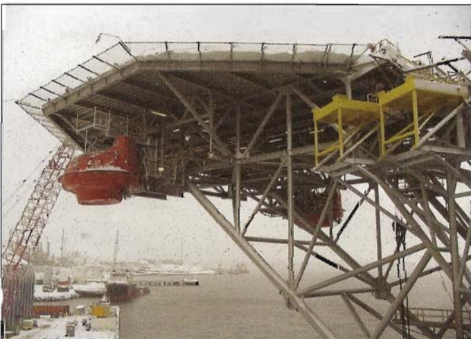
A view of the Halifax Harbour from just below the Global Santa-Fe's Galaxy II helipad. Note the orange lifeboat just below the helipad. Photo Courtesy of the Bercha Group.
